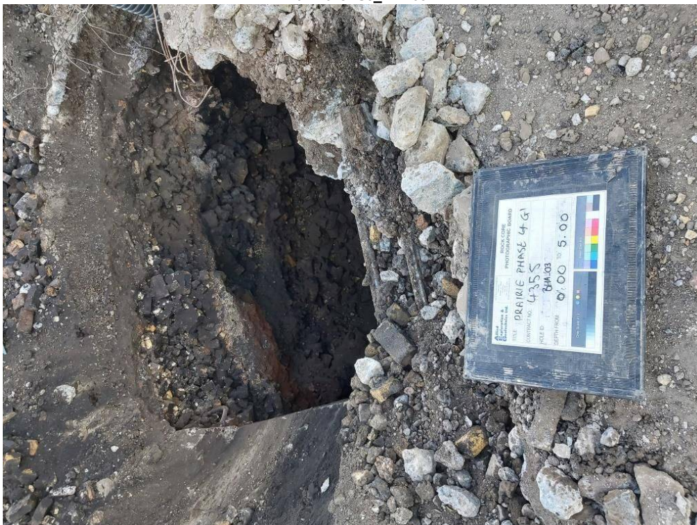
Figure S3_BHA03.2 Trial Pit for S3_BHA03
