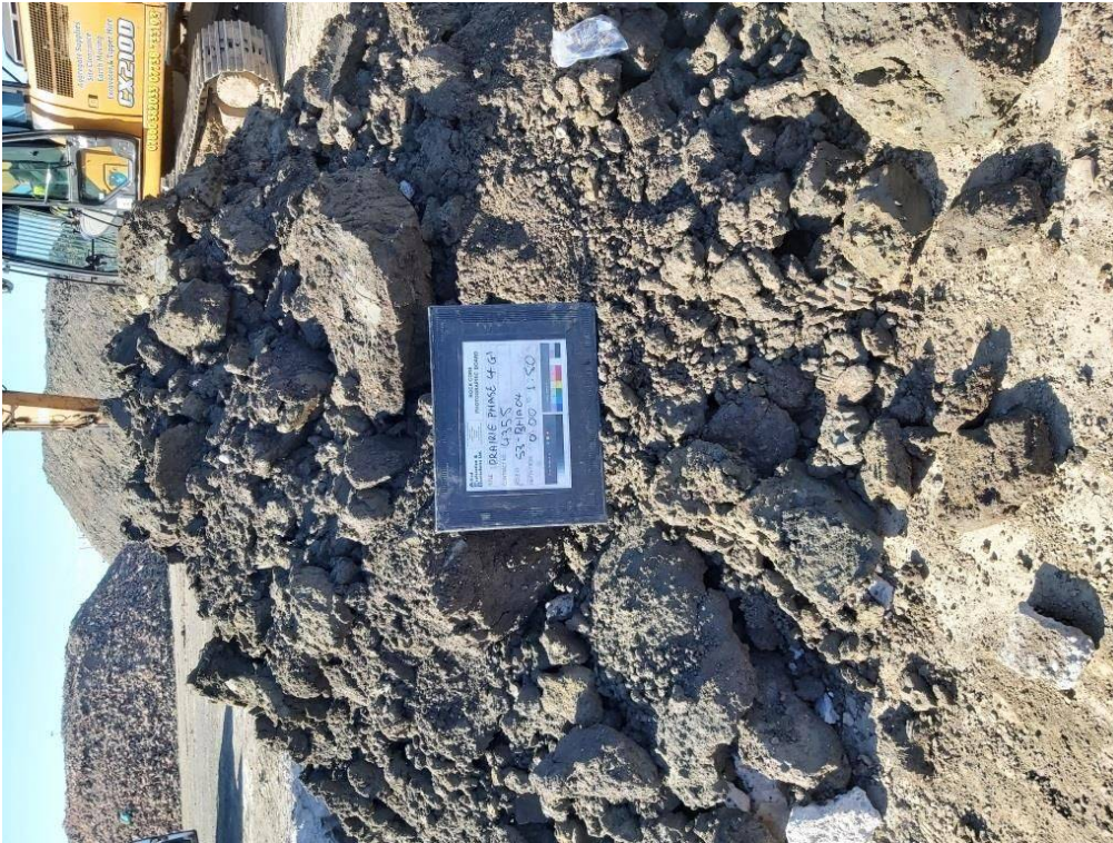
Figure S3_BHA04.3 Trial Pit for S3_BHA04
