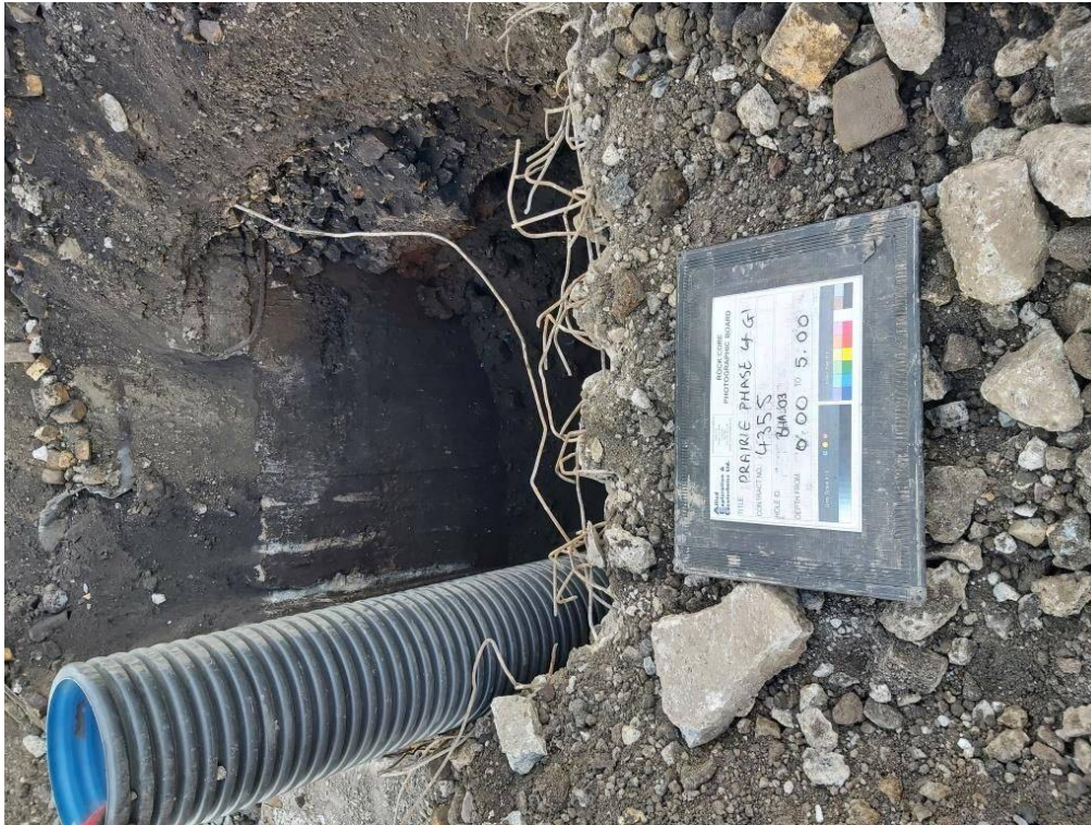
Figure S3_BHA03.1 Trial Pit for S3_BHA03
