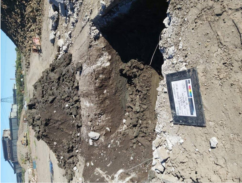
Figure S3_BHA04.1 Trial Pit for S3_BHA04
