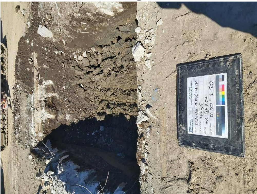
Figure S3_BHA04.2 Trial Pit for S3_BHA04
